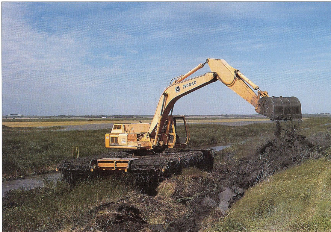
The backhoe has proven to be an effective cattail control tool, but it's slow compared to other methods. In addition to digging up the plants, a tool on the bucket can be used to cut cattail in flooded areas.
